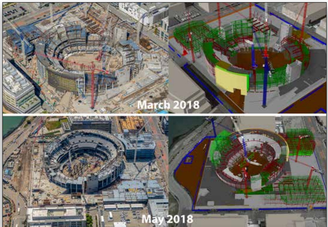
Using SYNCHRO for 4D visualization, Mortenson | Clark created 1,674 critical schedule activities with over 151,635 individual resource elements.
